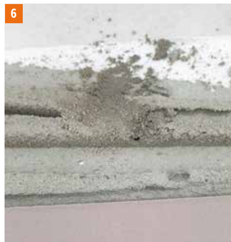
Photos 4, 5, 6 Geoflex Express. Hardness test of the adhesive mortar performed on the bonded „ridges” after 1.5 hours: strong pressure causes the mortar to crumble, the colour at the break is medium grey. The tiled surface can support load and grouting is already possible.
