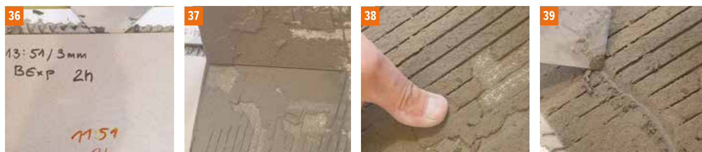
Photos 36, 37, 38, 39 Fast-setting adhesive no. 2 (class "F"). When the tile is lifted, it is obvious that the detachment occurred in the adhesive layer. The adhesive is only partially bonded and be easily rubbed off with a finger or tool.
